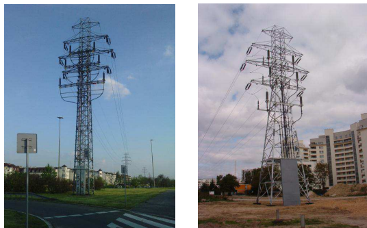
Figure 1. Transition towers of 110 kV overhead-underground transmission lines.
